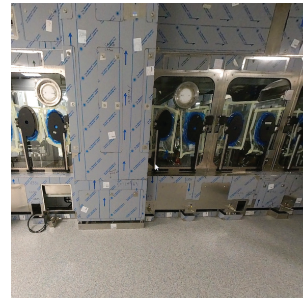
Installed equipment line with exposed base
