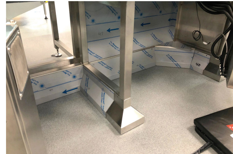
Installed skirting with removable access panels along bottom of the exposed equipment
